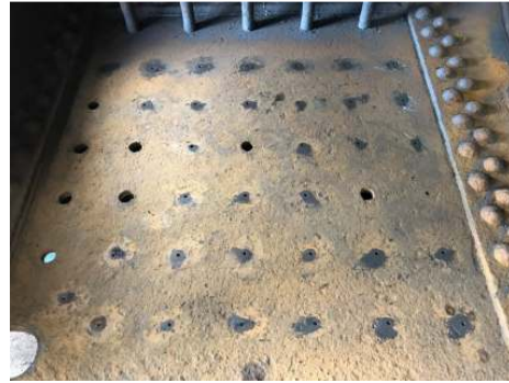
Figure 7 - Stays have been pilot drilled. Note the stays which have fallen out while needle gunning
