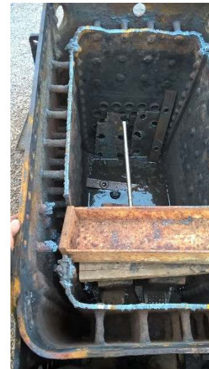
Figure 9 - Jacking bar used to remove the foundation ring. Note the stays haven’t been cut yet.
