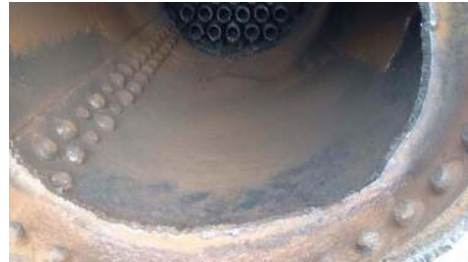
Figure 4 - Boiler barrel seam with 4 “screwed” repair rivets
