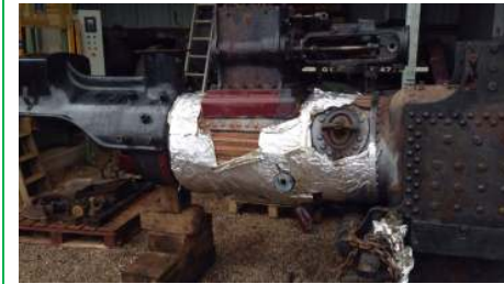
Figure 1 - Cladding sheets removed exposing tin foil wrapped boiler
