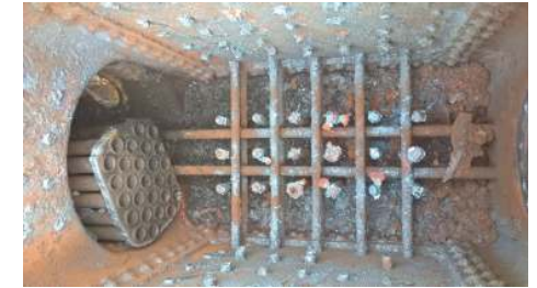
Figure 10 - Box removed showing cross stays. Note the tube nest pushed into barrel to aid box removal
