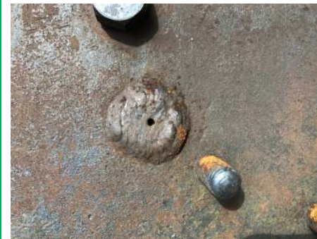
Figure 2 - Welded firebox stay, outside surface of hornplate
