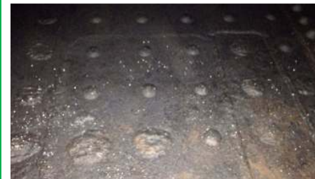
Figure 3 - Inside firebox showing plates "let-in" and welded stays
