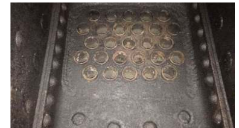
Figure 4 - Firebox tube nest cut out and welded back in, details to follow in Part 2
